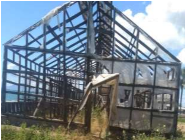
Figure 8 Damaged Community Solar Tent Drier at Malembo
