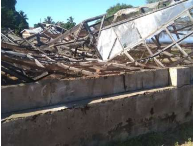
Figure 7 Damaged Solar Tent Drier at Lifuwu
